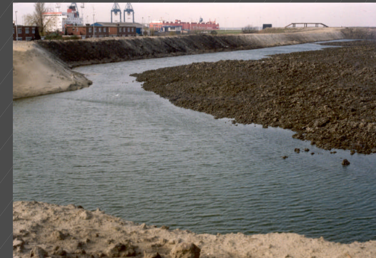
◀ Figure 3. Early stage in the construction of the test dike (November 1999). First a supportive sand dike is built (left). The confined zone is then filled with consolidated dredged material (right). The small community of Magershoek is visible in the top left corner. (Foto: verzameling Gemeentelijk Havenbedrijf - HB/TD).
